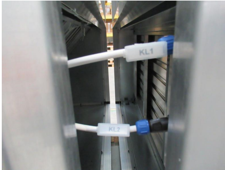
design of connectors on the border of the 1st and 2nd transport block - - power supply of ODA and EHA input damper actuators
